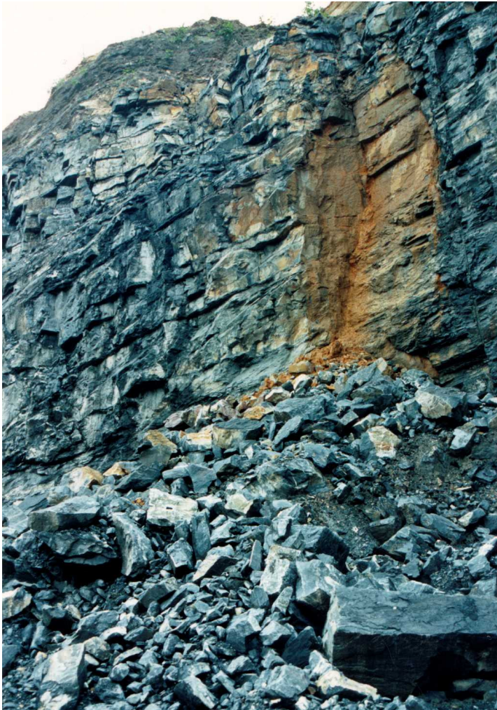
Figure 31: Structurally controlled failure in the face of a steep bench in a heavily jointed rock mass.
